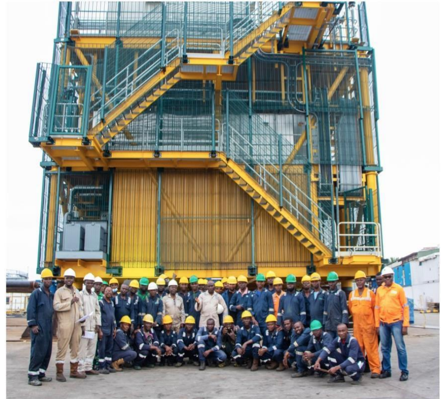
The construction of the MADU Conductor Supported Platform (CSP) for the development of MADU field of OML 85.
