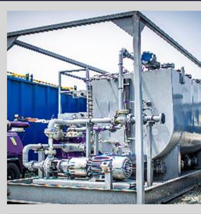
water treatment unit
