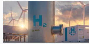
EPC Green Hydrogen Production Facility Canada. CM of the EPC phase of an electrolyzer plant incorporating Cummins electrolysis technology
