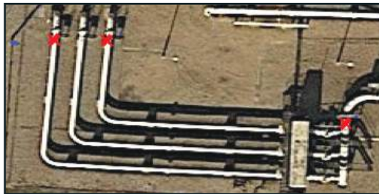
Leak locations confirmed
