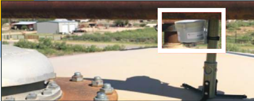
MethaneTrack™ endpoint mounted on tank near thief hatch
