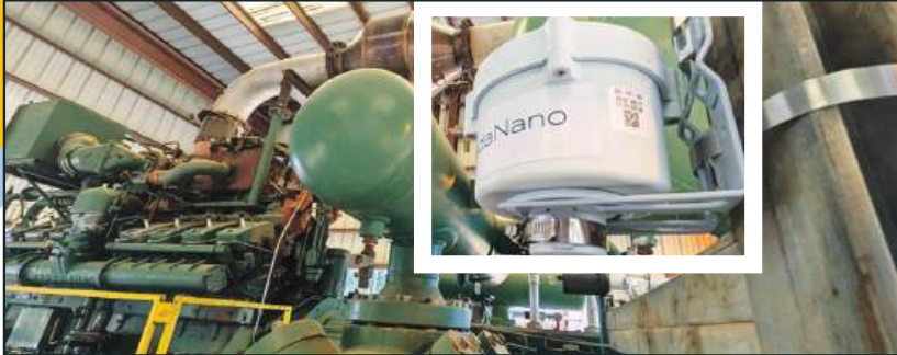
MethaneTrack™ endpoint mounted in close proximity to compressor
