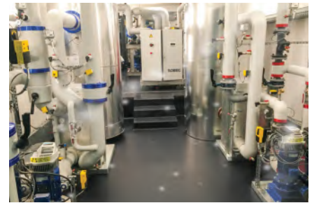
The technical room with the heat pump in the center.
