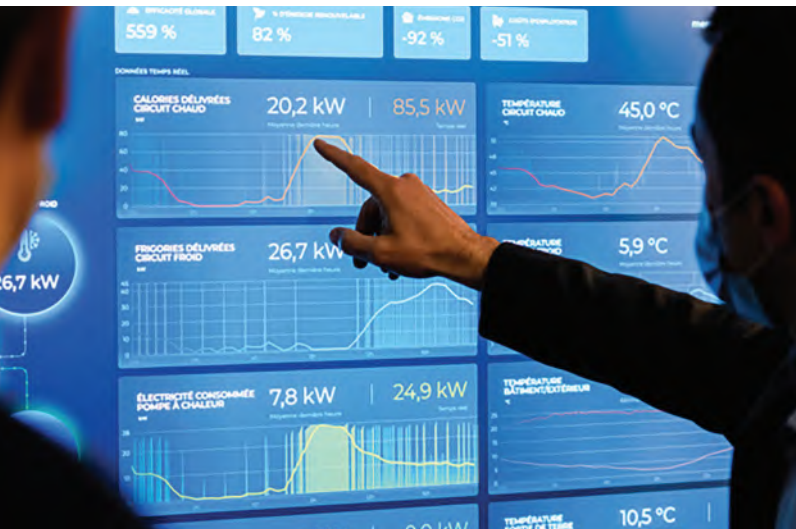
Dashboard view with principal parcels in over time of energy delivered (heating and cooling), electricity consumed and renewable underground energy produced.
