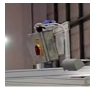
Mains Power Box & Cable Mounted Above Stand
