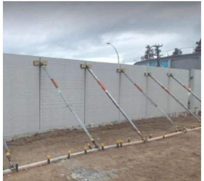
Holding wall in vertical position while it is set in place (Credit: QOROX Ltd.).
