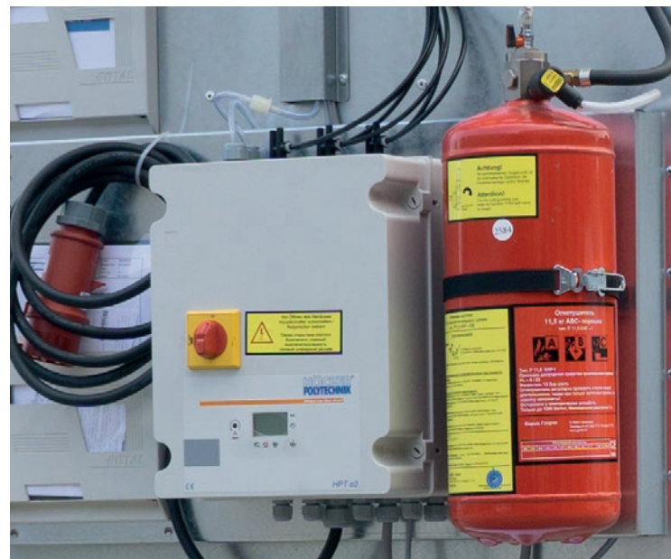
Fig. below: PLC-control, automatic fire extinguishing system
