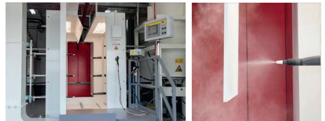
Modern powder coating plant for wood coating (Source: Karl Bubenhofer AG)
