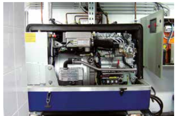
This three-phase Panda is installed in a basement. Main fuses, panel and radiator control are fitted in an electrical cabinet.
