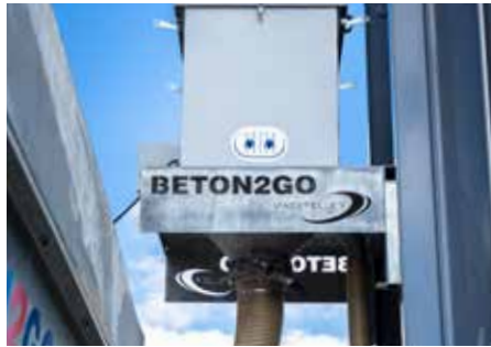
Cement dust filter
