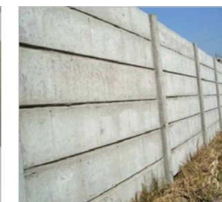
Pre-cast Compound Wall
