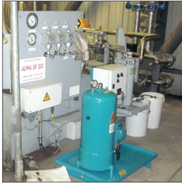
Gearbox, MAAG Gear with installation of a CJC® Fine Filter HDU 27/54 PV
