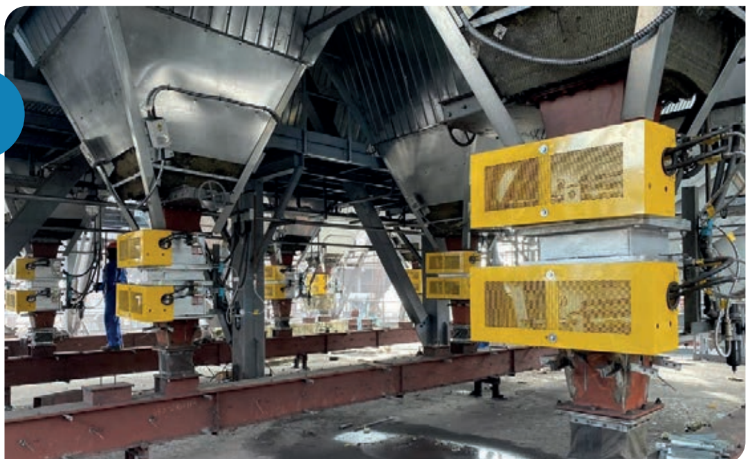
Plattco double-flap airlock valves on electrostatic precipitators at a cement plant in the US.
