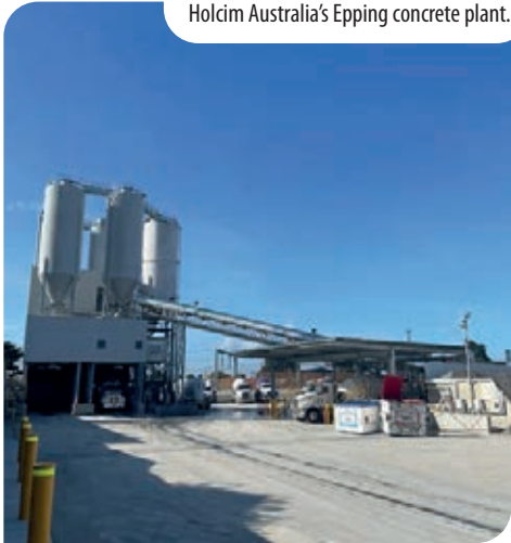
Holcim Australia's Epping concrete plant.
