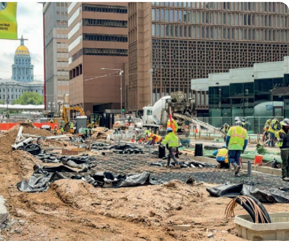
Workers preparing the ground for a concrete road base in Denver, Colorado. Credit: Ceri Breeze via Shutterstock.
