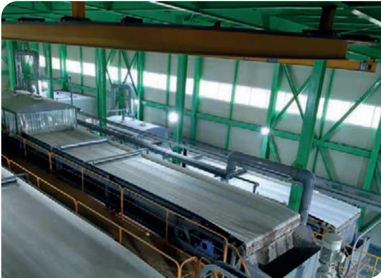
Figure 5: Vacuum belt filters with multi-stage washing for separating the dust from the brine.
