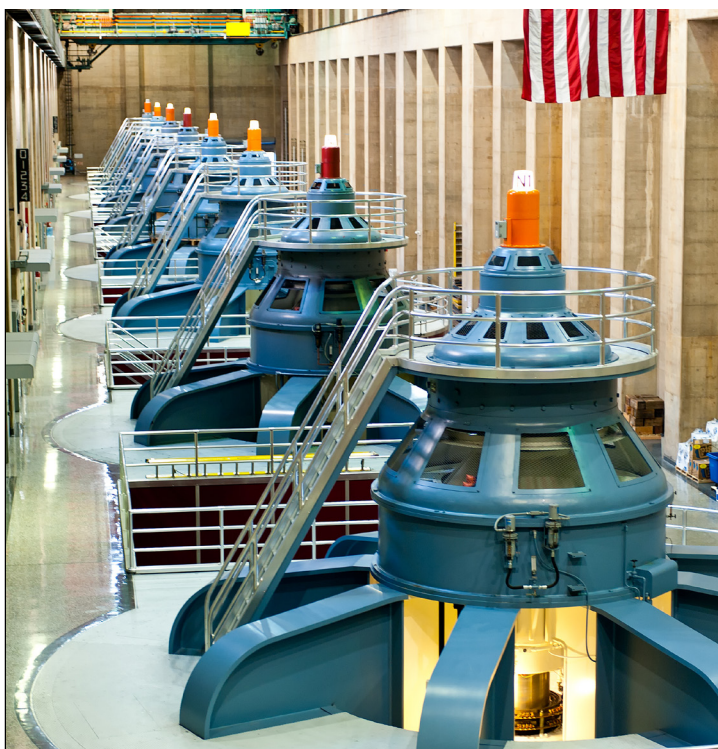
Turbines and generators at the Hoover Dam hydroelectric plant on the Colorado River, USA.
