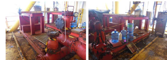
Location: Module 2 Lower Deck Remarks: Both firewater pump P-210A/B were removed.
