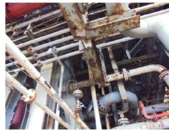
Location: Lower Deck Module 2 Remarks: Area was congested with piping and xmas tree.
