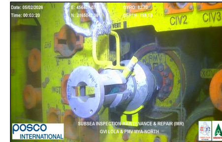
< LOLA As-left Inspection >
