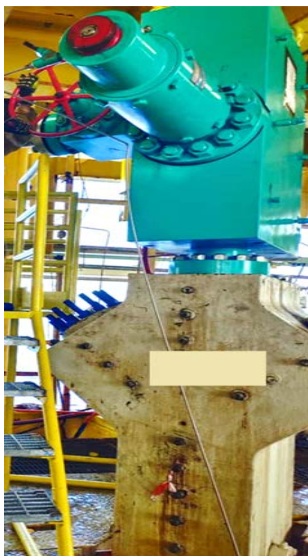
Fig. 2—Completed installation of new Xmas tree on top of existing tree due to difficulties to remove the corroded existing tree and high risk of leaking due to unknown flange connection
