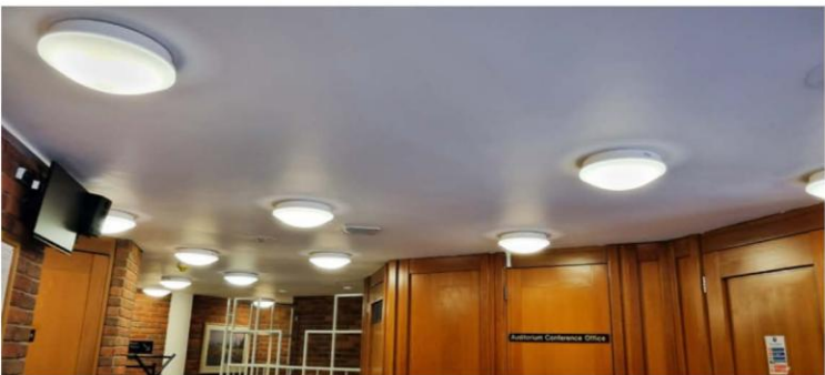
A proliferation of modern lighting in the Auditorium foyer
