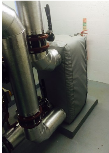
Figure 5.5.2: Separating Plate Heat Exchanger (with isolation valves)
