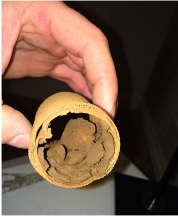
Figure A6.1.1: Contaminated Lateral Strainer
