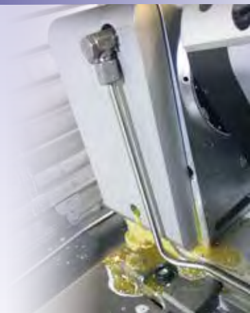
severe oil loss
